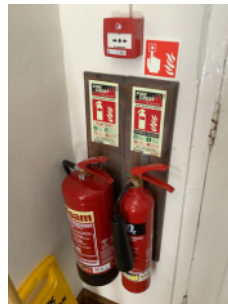
Kitchen fire point
