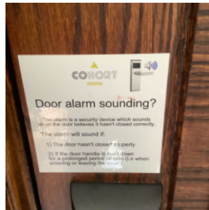
Door alarm to room exit door.
